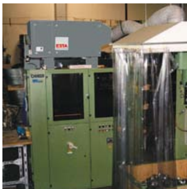
Oil Mist Separator in operation
